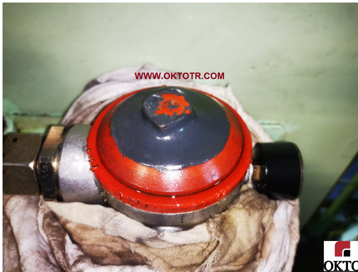
BROKEN FILTER COVERS
